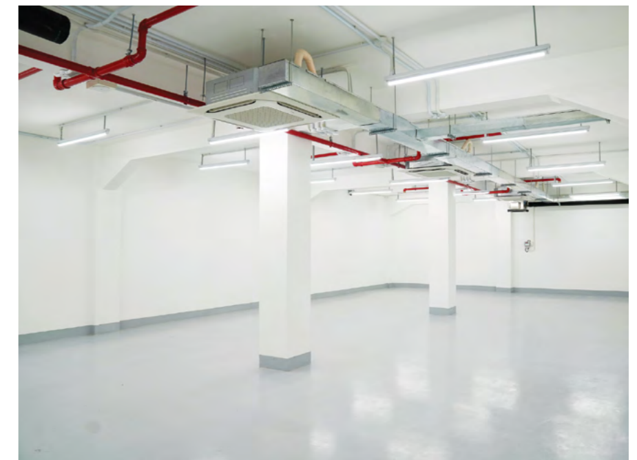
▶ Outfitting of the new archive repository nears completion, seen here awaiting assembly of compact shelves.
