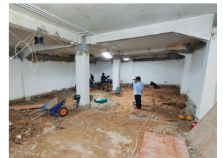
▶ Former office space is converted into a state-of-the-art archive repository. Note the ground reinforcement in progress.
